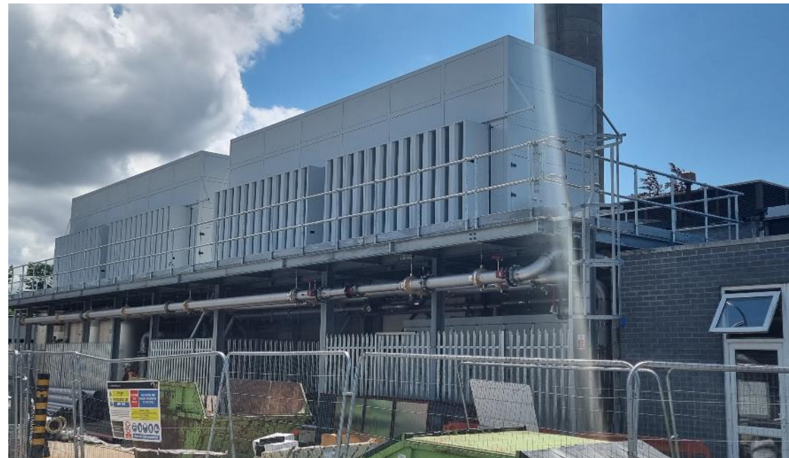
Two heat pumps were fitted to our Combined Heat and Power plant in 2024, which will save around 4,000t of CO 2 e annually. This was part of the Public Sector Decarbonisation Scheme.
